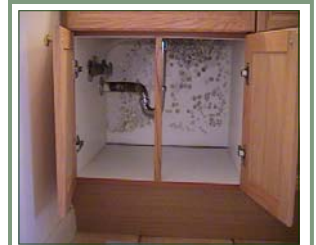
Common places for mold growth include storage space underneath sinks.
