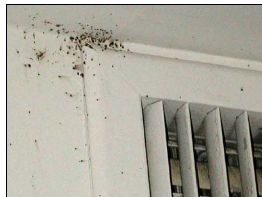
Bed bug fecal stains near a duct indicate harborage and possible movement. Photo by R. Cooper.
