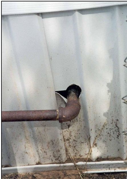
Figure 7. Rodent entry around pipe
