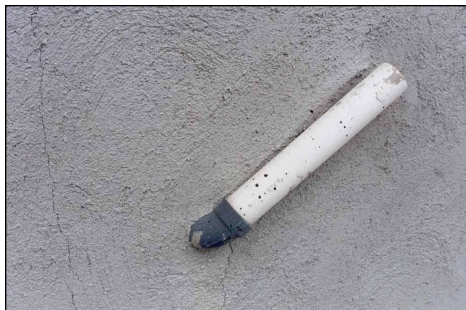
Figure 8. Pipe well sealed with cement to prevent rodent entry
