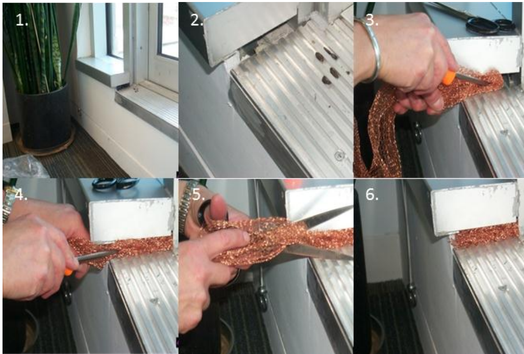
Figure 38: Steps for installing copper mesh to exclude rodents: fecal pellets (droppings) were detected, area was cleaned with bleach, and snap traps were set. Stuf-Fit® copper mesh was installed to eliminate rodent access point. Figure credit: NPS Figure.
