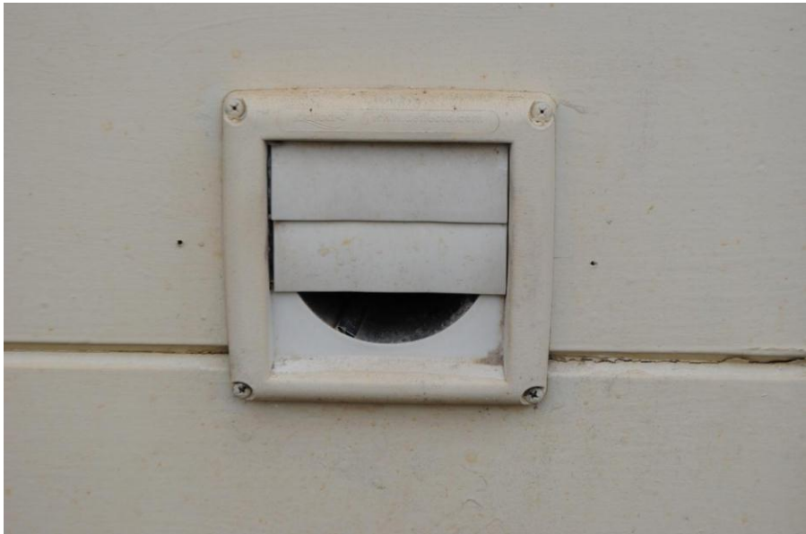
Figure 5: The lower exhaust flap on this dryer vent is missing and provides rodents access to the building interior. A new rodent proof flap needs to be installed with ¼ inch hardware cloth to exclude rodents. The vent must also be periodically cleaned to prevent lint build up. Figure credit: NPS Figure.
