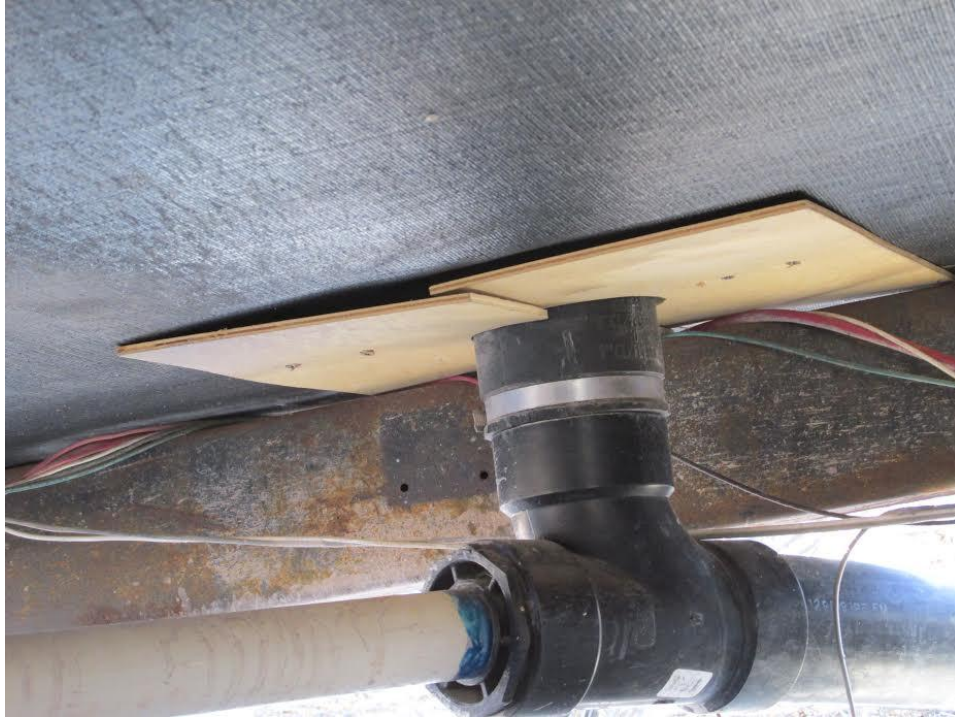
Figure 28: The underside of trailers should be rodent proofed prior to human occupation. Figure credit: NPS Figure.
