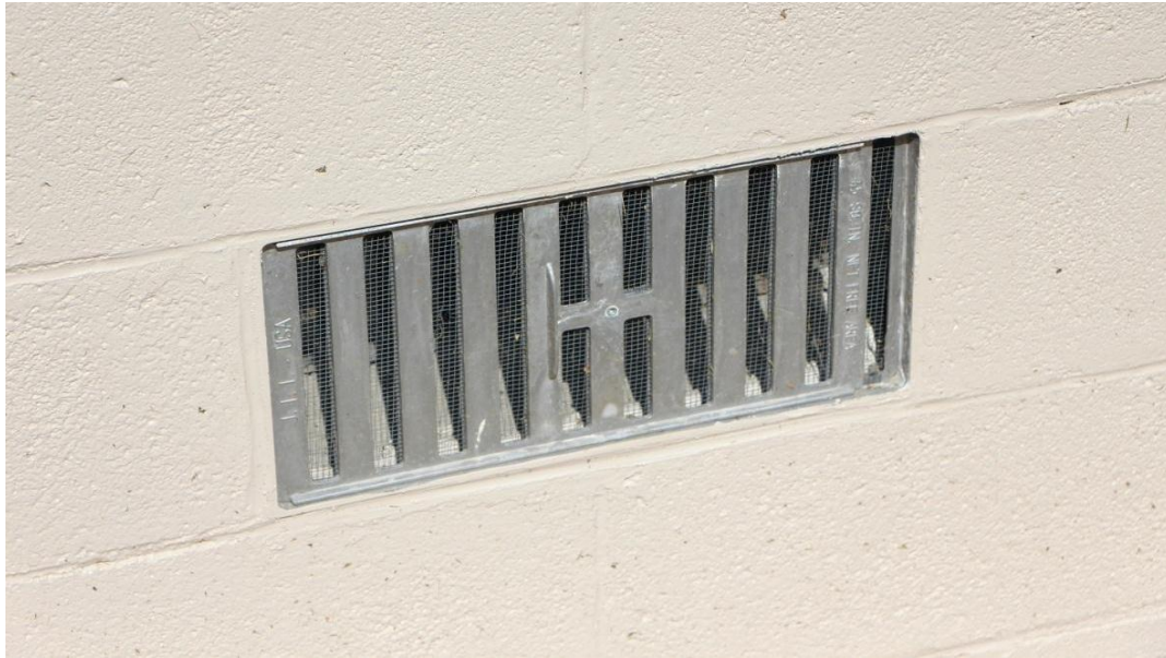
Figure 7: This crawl space vent is properly screened with ¼" hardware cloth (visible behind the metal bars). Figure credit: NPS Figure.
