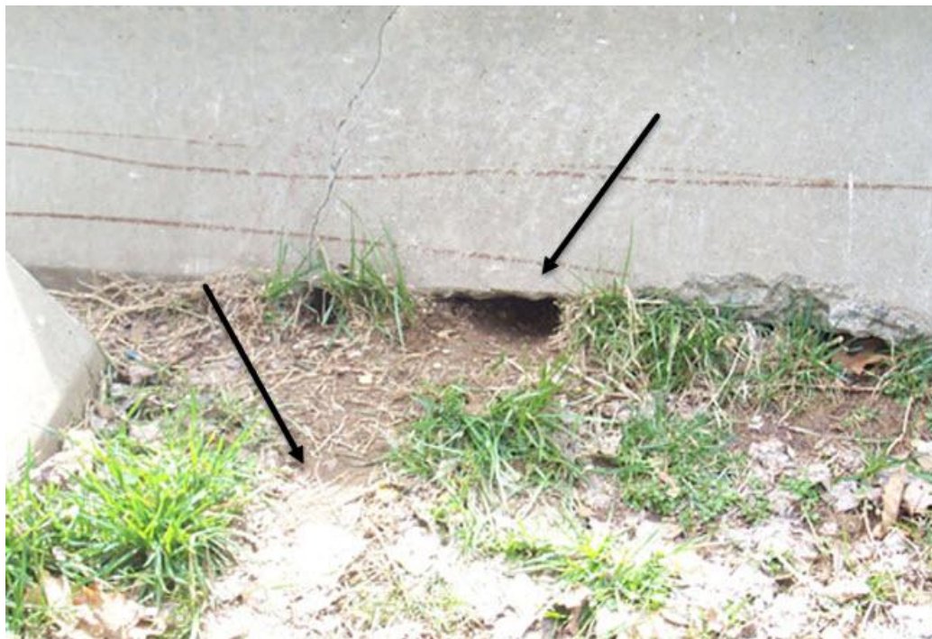
Figure 28: This active rodent burrow is located at the foundation of the building. Note the entrance and runway is clear of vegetation and the rodent has created a “run”. Figure credit: NPS Figure.
