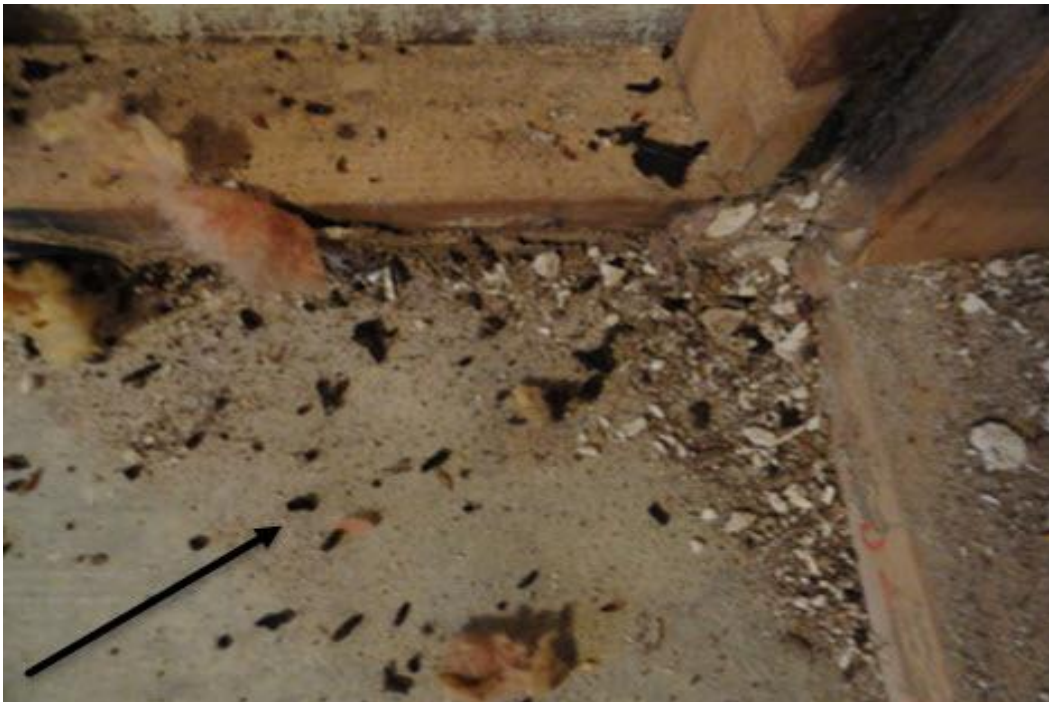
Figure 18: Rodent feces (droppings) confirm rodent activity in this wall void. Figure credit: Carol DiSalvo.
