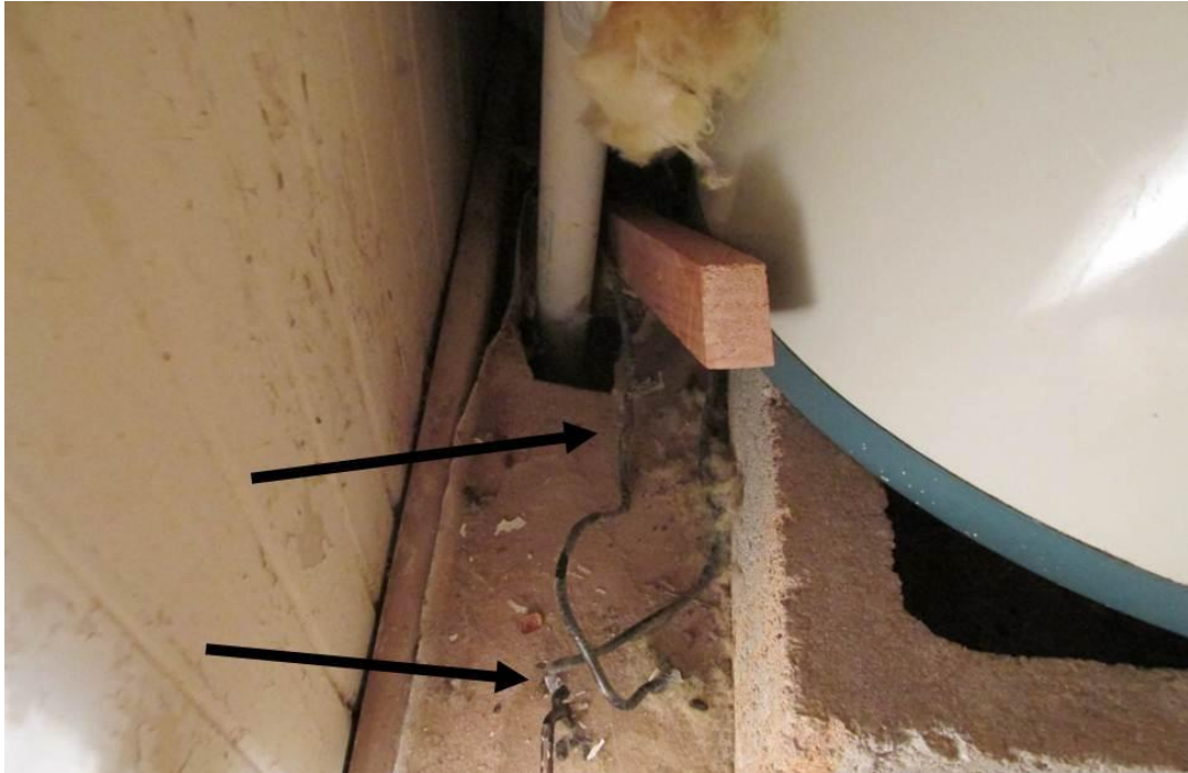
Figure 20: Wire damage from packrats. Figure credit: Charles Conner.
