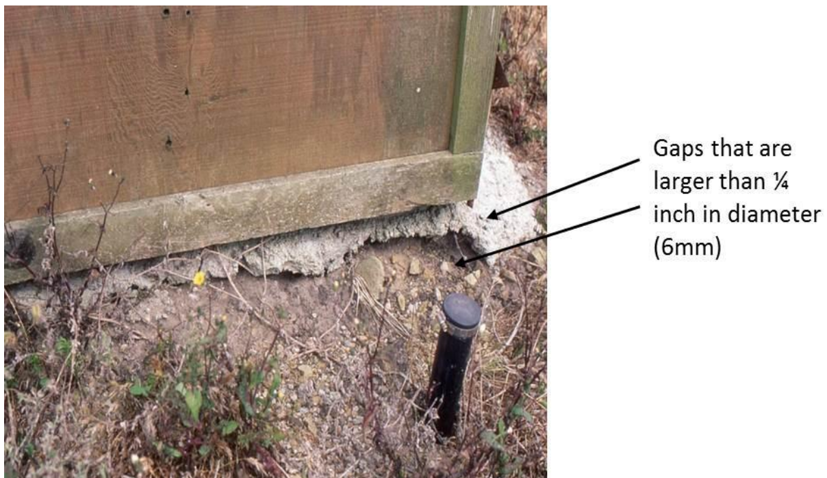
Figure 6: This foundation has a gap between the foundation and building providing potential rodent access into the building. Figure credit: NPS Figure.
