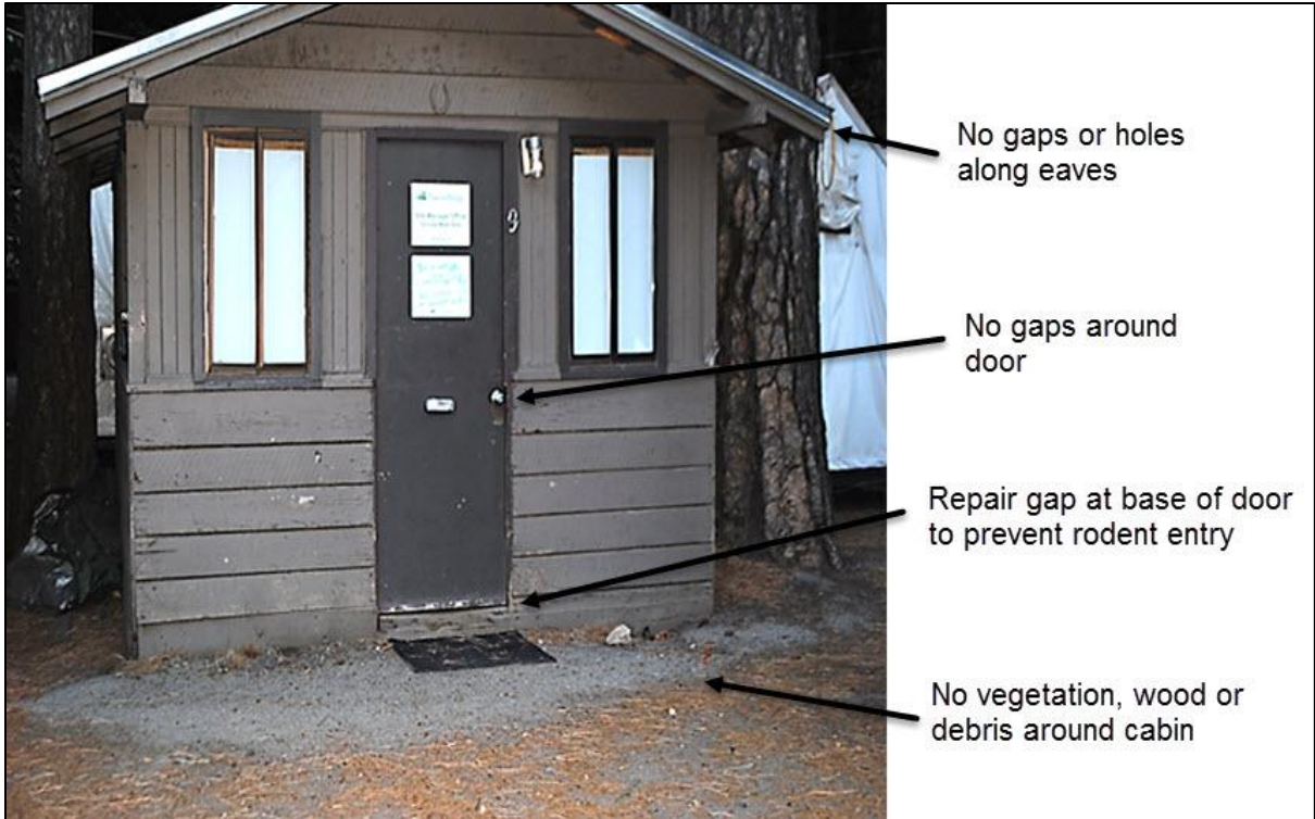
Figure 4: Additional points to evaluate on a cabin include gaps around eaves or door and the presence of vegetation, wood, or other debris around the foundation of the cabin. Figure credit: Bruce Badzik.
