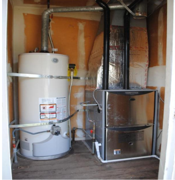
Figure 17: Evaluate utilities for potential entry points, which are commonly found behind the hot water heater or furnace. Also check for nesting material underneath or behind these appliances. Figure credit: Bruce Badzik.
