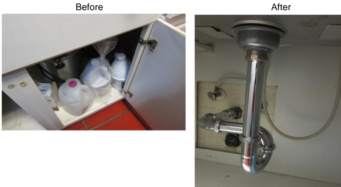
Figure 5. Before and after Cleaning, Clean Room Sink
