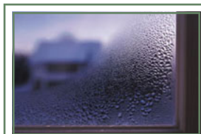
Condensation on windows is a sign of excess moisture.
