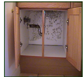
Common places for mold growth are cabinets under sinks, often due to pipe leaks.
