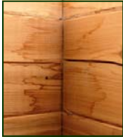
Signs of leaks include water stains on walls, ceilings and floorboards.
